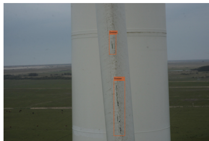
(a) Erosion in the LE, leading to degradation of the gel coat
