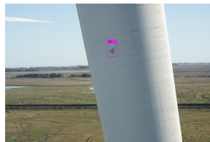
(f) Receptor partially covered by top coat and with a crack on sealant around it
