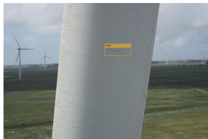
(c) Longitudinal Crack
